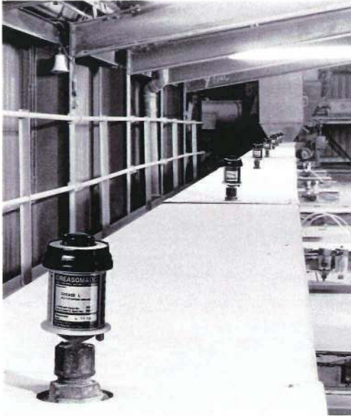
• feed mill screw conveyors
